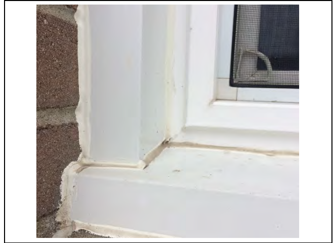
Photo 2: Presumed asbestos-containing exterior window caulking at Unit F.
