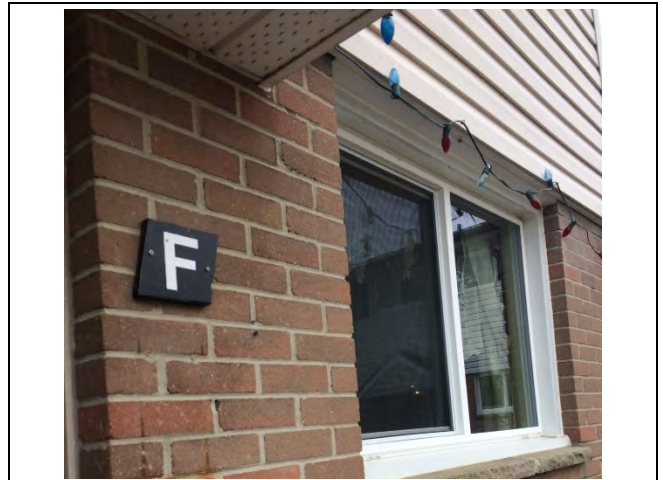
Photo 4: Presumed asbestos-containing brick mortar was observed on exterior walls at Unit F.
