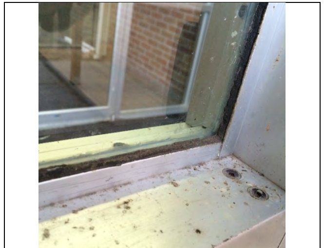
Photo 8: Exterior window glazing compound presumed to be asbestos-containing.
