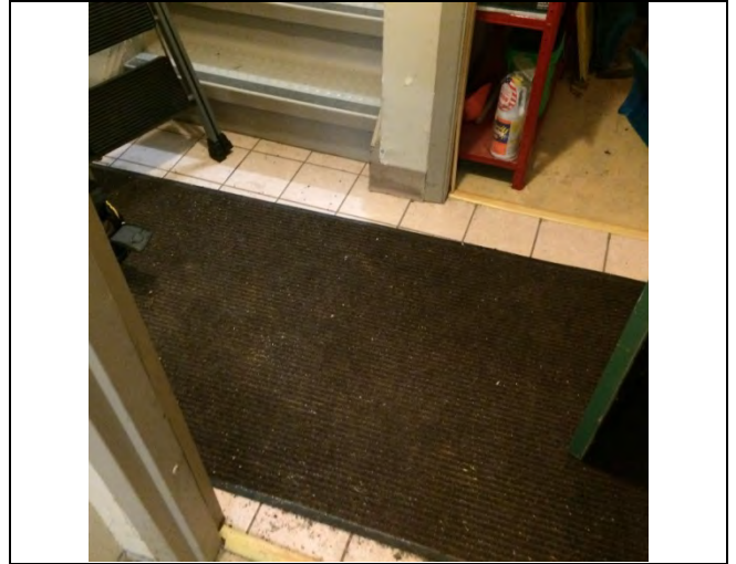
Photo 6: Ceramic tile grout presumed to be asbestos-containing in the back door entrance.
