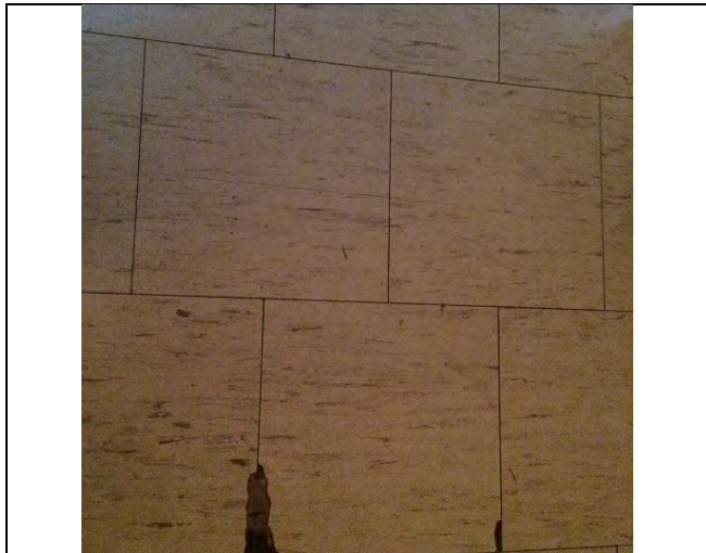
Photo 3: 12"x12" vinyl floor tile – beige with brown streaks identified to be asbestos-containing in Unit 201 (0.77% Chrysotile).
