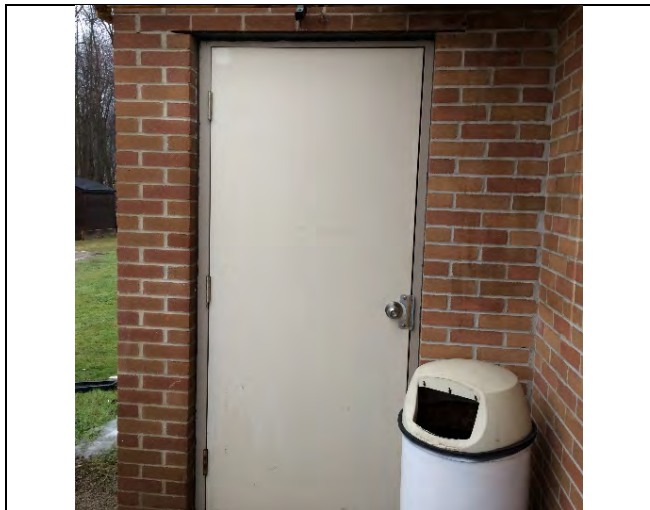
Photo 7: Exterior door caulking and brick mortar presumed to be asbestos-containing.
