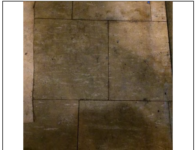
Photo 4: 12"x12" vinyl floor tile – grey with brown streaks identified to be asbestos-containing in Unit 201 (1.44% Chrysotile).
