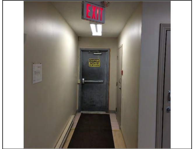
Photo 2: Drywall joint-fill compound identified to be asbestos-containing in the hallway (1% Chrysotile). Fire rated doors is presumed to be asbestos-containing.
