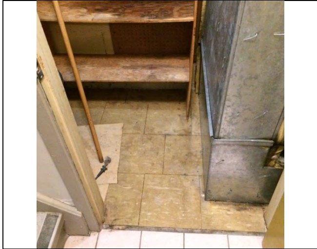
Photo 5: 12"x12" vinyl floor tile – yellow with white streaks identified to be asbestos-containing in the west storage room (0.77% Chrysotile).
