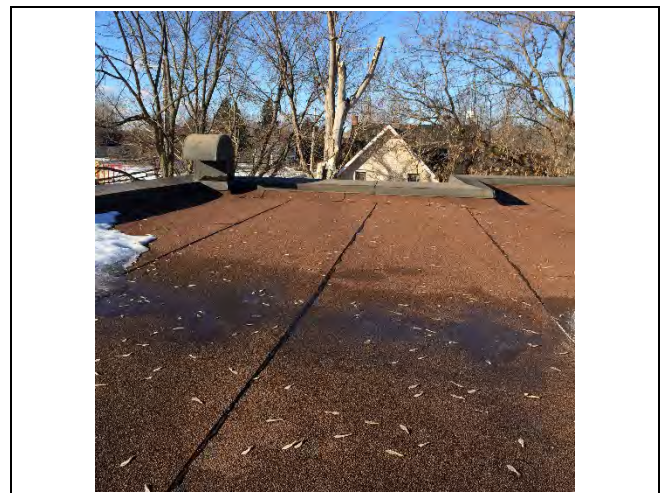
Photo 8: Roof shingles are presumed to be asbestos-containing.
