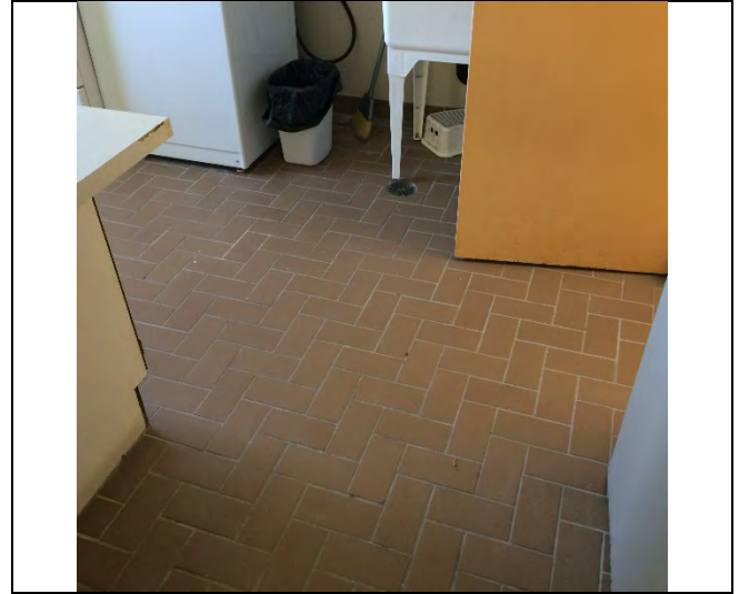
Photo 6: Ceramic tile grout and mortar/adhesive is presumed to be asbestos-containing in the laundry room.
