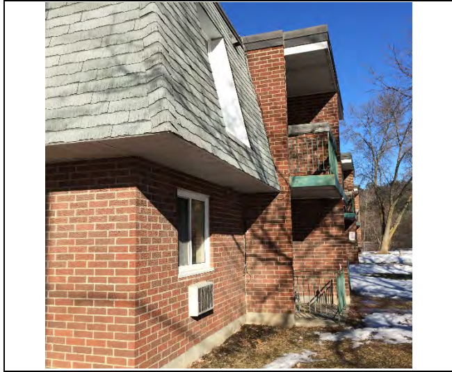
Photo 5: Brick mortar is presumed to be asbestos-containing.
