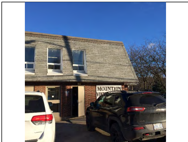
Photo 7: Exterior window and door caulking is presumed to be asbestos-containing.
