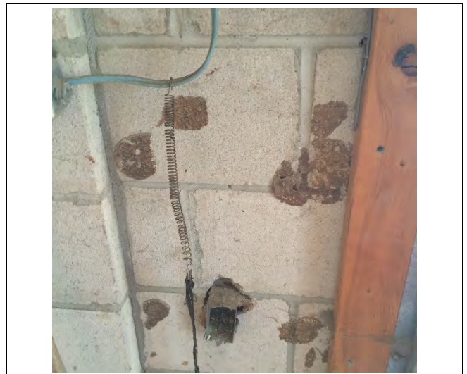
Photo 4: Mastic puck – brown on the block walls in the exterior garage identified to be asbestos-containing (1.2% Chrysotile).
