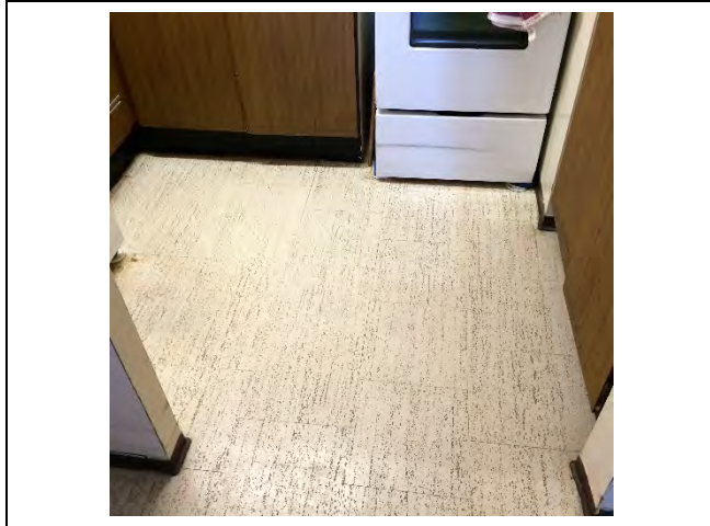
Photo 1: 12"x12" vinyl floor tile – beige with grey specks identified to be asbestos-containing in Unit 101 (1.45% Chrysotile).
