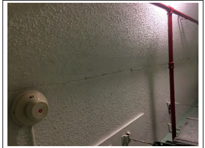
Photo 2: Asbestos-containing texture material observed to be cracking in the 2 nd floor laundry room ceiling.
