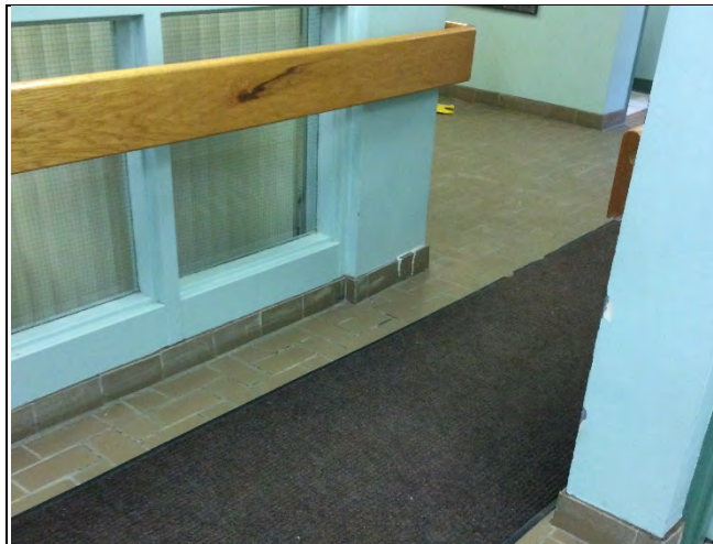
Photo 3: Asbestos-containing drywall joint-fill compound on the walls and presumed asbestos-containing ceramic tile grout and mortar/adhesive on baseboards and floor observed to be in good condition in the 1 st floor corridor.
