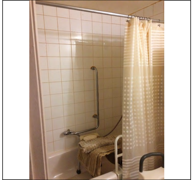
Photo 6: Presumed asbestos-containing ceramic tile grout and mortar/adhesive observed to be in good condition on walls in the washroom at unit 103.
