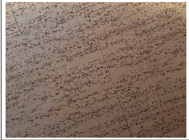
Photo 1: Asbestos-containing 12"x12" vinyl floor tiles – beige with dots (2.24% Chrysotile) in unit 103 hallway.
