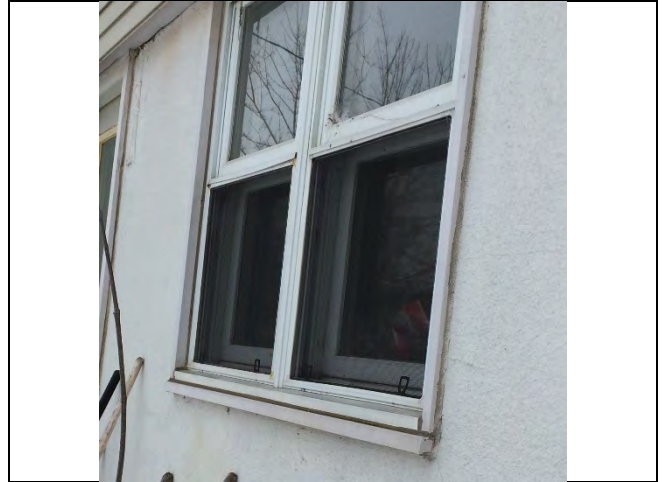
Photo 2: Presumed asbestos-containing exterior window caulking – beige on the exterior back window.
