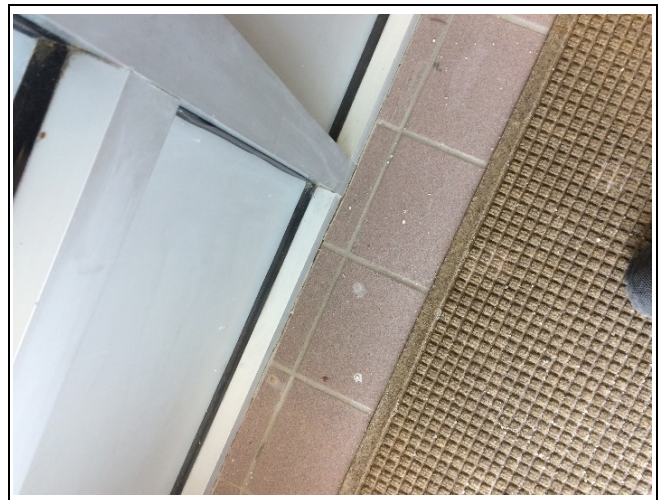
Photo 4: Presumed asbestos-containing ceramic tile grout and mortar/adhesive at the main entrance.
