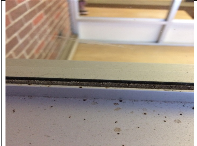
Photo 5: Asbestos-containing exterior window glaze – white observed to be in good condition on the windows at the main entrance doors.
