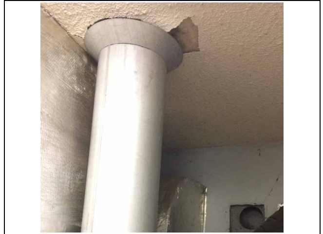
Photo 2: Asbestos-containing texture coat observed to be in poor condition on the ceiling in the storage by unit 214.
