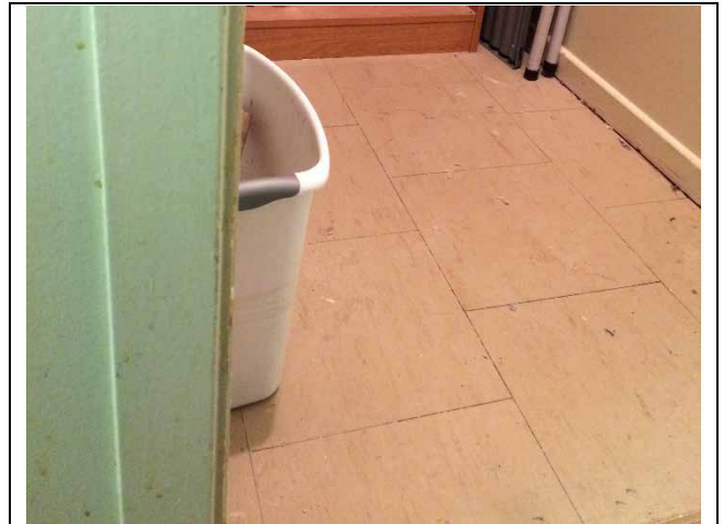
Photo 4: Asbestos-containing 12"x12" vinyl floor tiles – beige with light brown smears observed to be in good condition in unit 213 closet.
