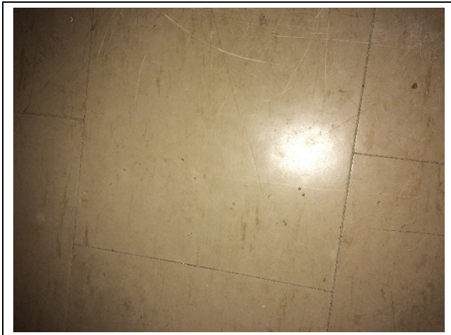
Photo 3: Asbestos-containing 12"x12" vinyl floor tiles – brown with brown streaks observed to be in good condition in unit 103 bedroom.
