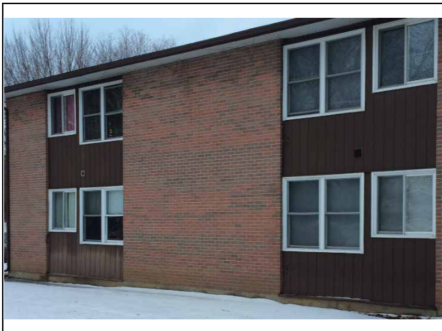
Photo 7: Presumed asbestos-containing brick mortar observed to be in good condition on the North exterior walls.
