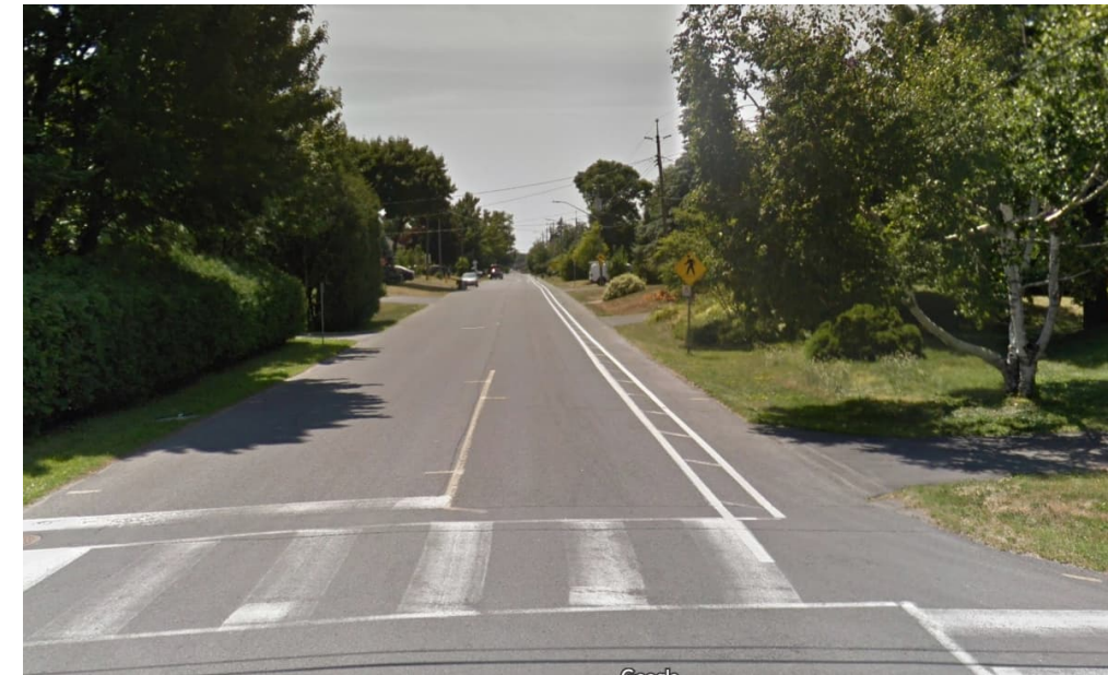
Figure D-5: A buffered paved shoulder on a residential street in Ottawa intended for use by pedestrians and cyclists
