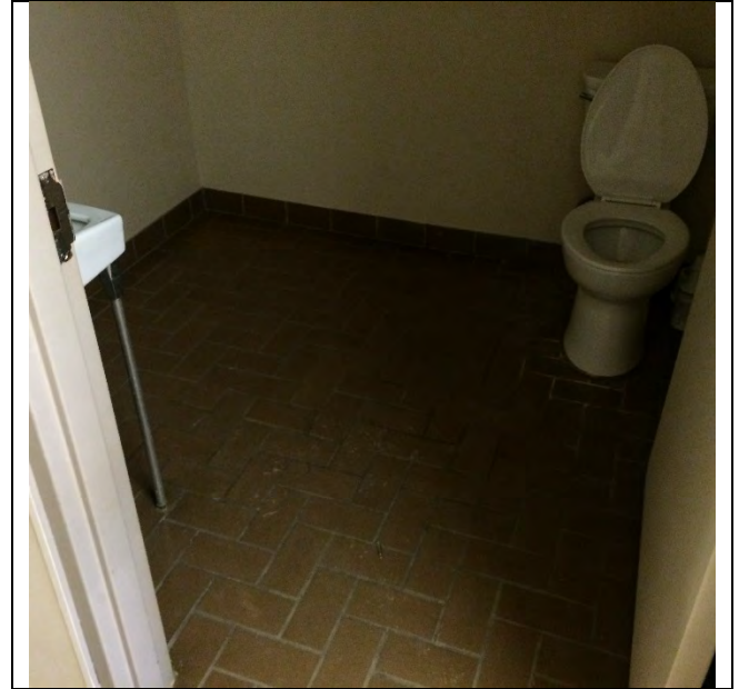
Photo 6: Ceramic tile grout and mortar/adhesive are presumed to be asbestos-containing in the washroom.
