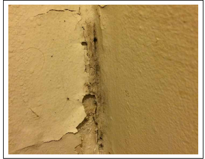
Photo 2: Asbestos-containing drywall joint-fill compound observed to be in poor condition on the wall in the foyer at 280 Bartholomew Street Unit #4.
