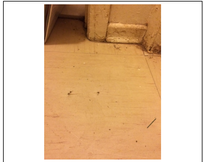
Photo 4: Asbestos-containing 12"x12" vinyl floor tiles – beige with brown streaks observed to be in good condition on the basement landing at 280 Bartholomew Street Unit #4.
