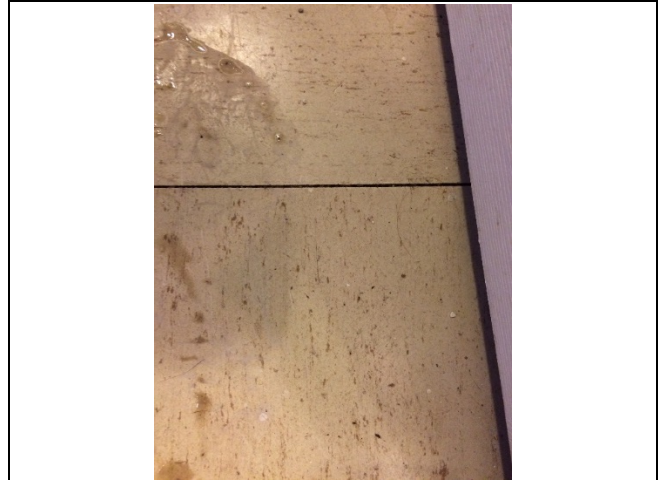
Photo 6: Asbestos-containing 12"x12" vinyl floor tiles – beige with black flecks observed to be in good condition on the basement landing at 280 Bartholomew Street Unit #8.
