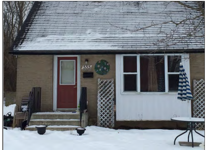
Photo 4: Presumed asbestos-containing brick mortar, roofing materials, and roof caulking.
