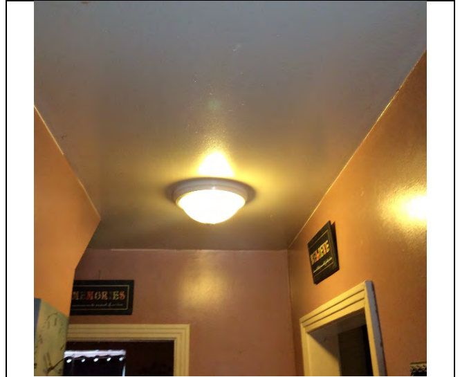
Photo 2: Asbestos-containing drywall joint-fill compound (1% Chrysotile).
