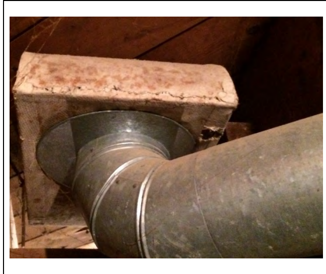
Photo 1: Asbestos-containing duct insulation paper wrap (60% Chrysotile) in poor condition.
