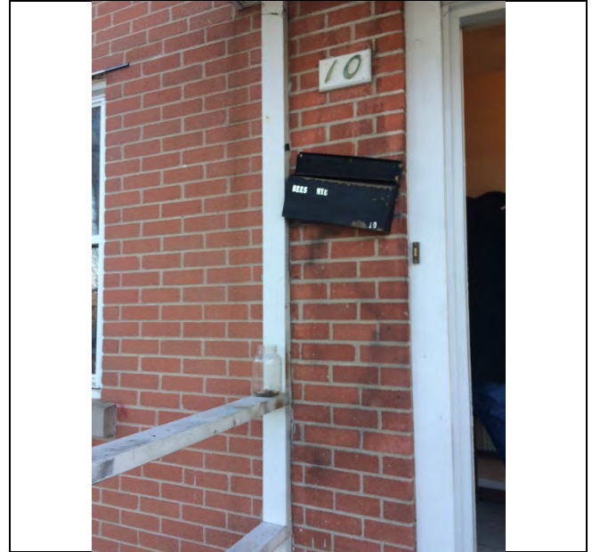
Photo 2: Presumed asbestos-containing brick mortar and exterior door caulking – white observed on the exterior.
