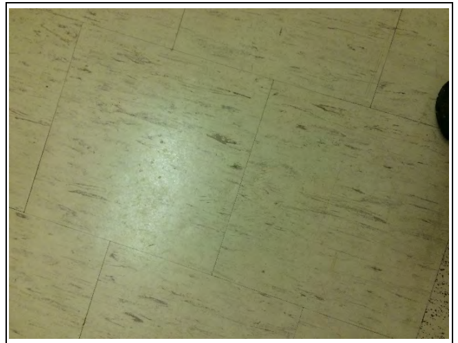
Photo 8: Asbestos-containing 12"x12" vinyl floor tile – beige with brown.
