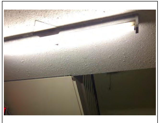
Photo 4: Asbestos-containing texture coat in the 1 st floor north stairs.
