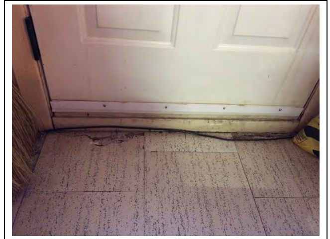
Photo 2: Asbestos-containing 12"x12" vinyl floor tile – beige with black dots observed to be in poor condition (cracked tiles) in the living room of Unit 108.
