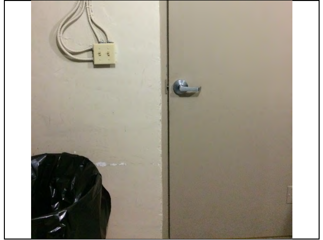
Photo 6: Asbestos-containing plaster observed in the garbage room.
