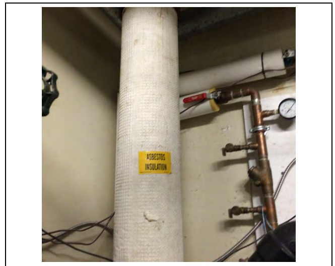
Photo 4: Cement pipe presumed to be asbestos-containing in the mechanical room.
