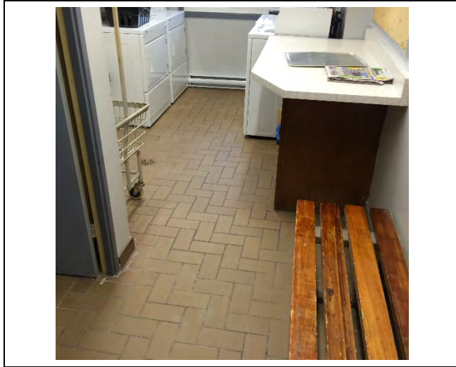
Photo 5: Ceramic tile grout and mortar/adhesive presumed to be asbestos-containing.
