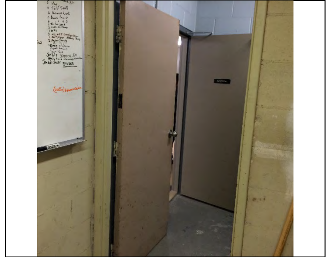
Photo 6: Fire rated doors – metal, presumed to be asbestos-containing.
