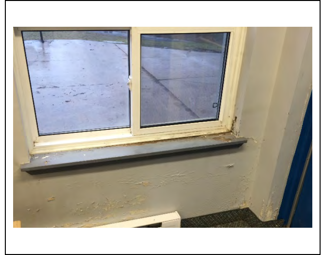
Photo 2: Asbestos-containing drywall joint-fill compound (1% Chrysotile) observed to be damaged in the lounge.
