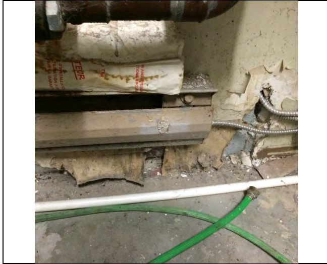
Photo 1: Asbestos-containing drywall joint-fill compound (1% Chrysotile) observed to be damaged in the mechanical room.
