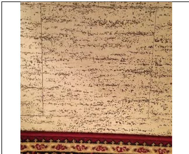
Photo 3: 12"x12" vinyl floor tile – beige with grey specks identified to be asbestos-containing (4.08% Chrysotile).
