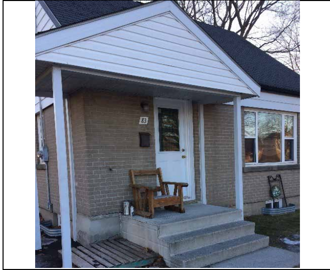
Photo 9: Presumed asbestos-containing exterior window and door caulking – white and brick mortar at the front exterior of 83 Brighton.
