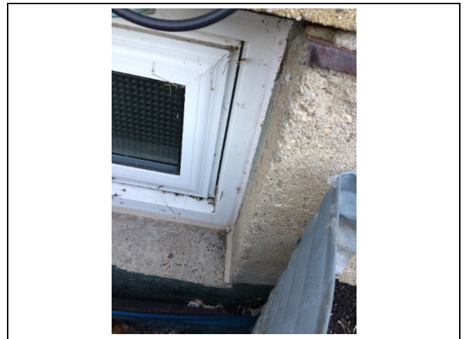
Photo 8: Presumed asbestos-containing exterior caulking – white on a basement window of 43 Brighton Crescent.
