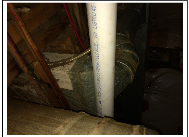
Photo 2: Asbestos-containing duct insulation paper wrap (70% Chrysotile) in the basement of 116 Brighton Crescent.
