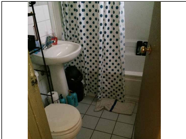
Photo 7: Presumed asbestos-containing ceramic tile grout and mortar/adhesive on the washroom walls and floor of 43 Brighton Crescent.
