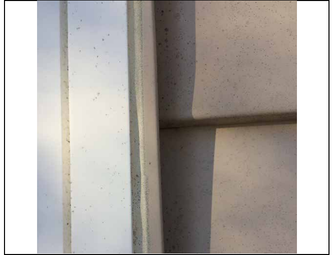
Photo 14: Presumed asbestos-containing exterior window caulking - white at the side window of 84 Brighton.
