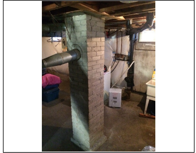
Photo 6: Presumed asbestos-containing brick mortar on a column in the basement of 43 Brighton Crescent.
