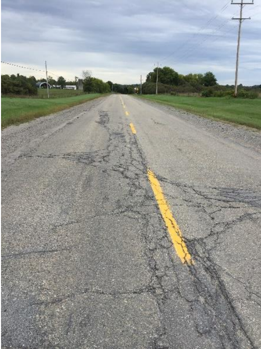
Poor (40 to 60 PCI)
