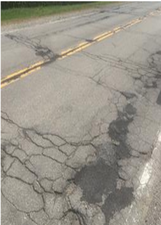
Very Poor (<40 PCI)
