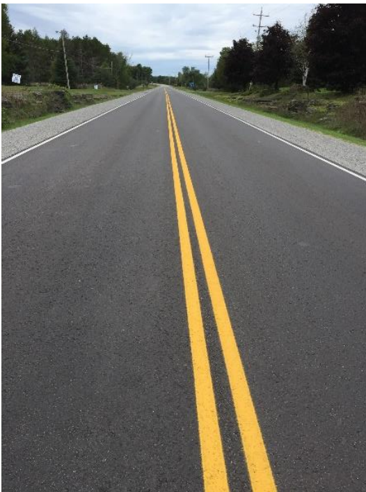
Figure 3-2: Road Condition Examples
