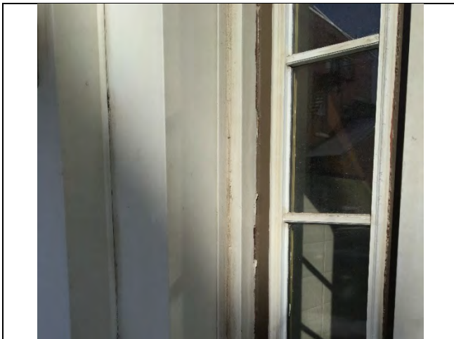
Photo 3: Presumed asbestos-containing exterior door caulking – white observed at 201 Prescott Street.
