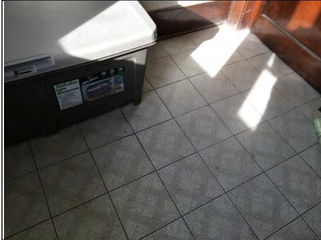
Photo 1: Presumed asbestos-containing ceramic tile grout and mortar/adhesive observed in unit 6 at 201 Prescott Street.
