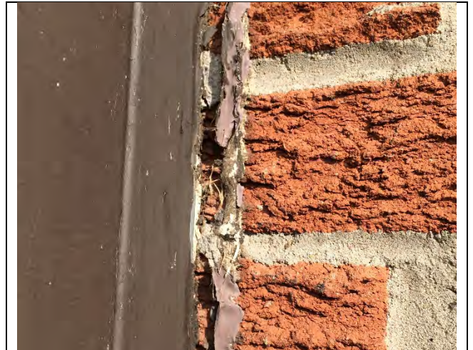
Photo 4: Asbestos-containing exterior door caulking – white was observed beneath brown caulking at the exterior west stairwell.
