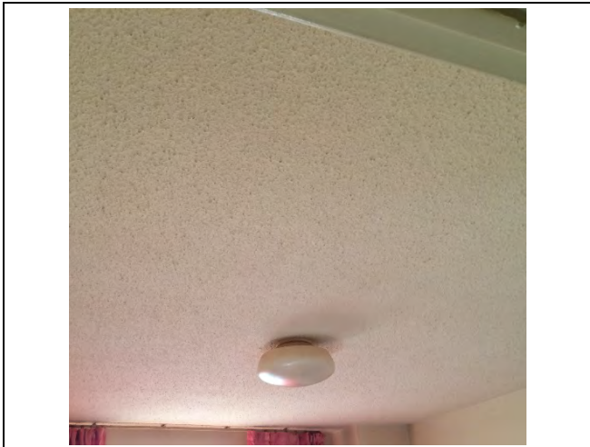
Photo 3: Asbestos-containing stucco on ceiling was observed in unit 107.
