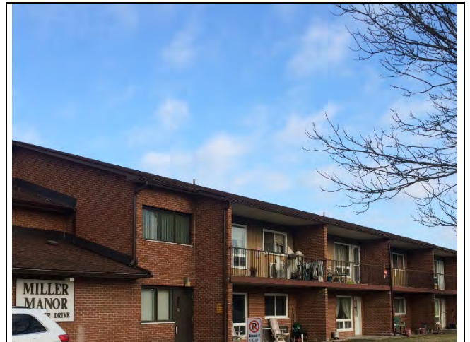
Photo 8: Presumed asbestos-containing brick mortar observed on exterior walls
