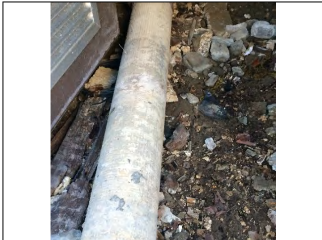
Photo 7: Presumed asbestos-containing cement pipe was observed in the crawlspace.
