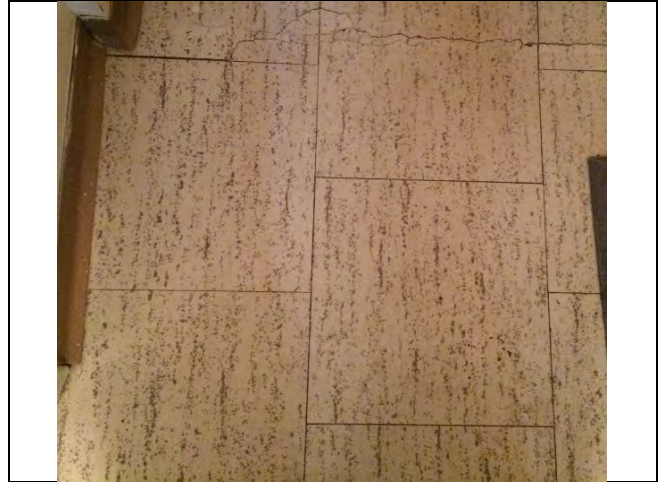
Photo 2: Asbestos-containing 12"x12" vinyl floor tile – beige with grey specks was observed in unit 209 hallway.
