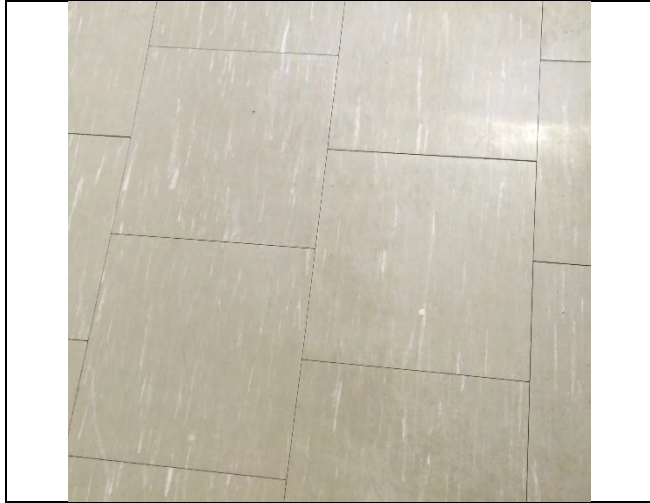
Photo 5: Asbestos-containing 12"x12" vinyl floor tile – olive with white streaks was observed in the east stairwell.
