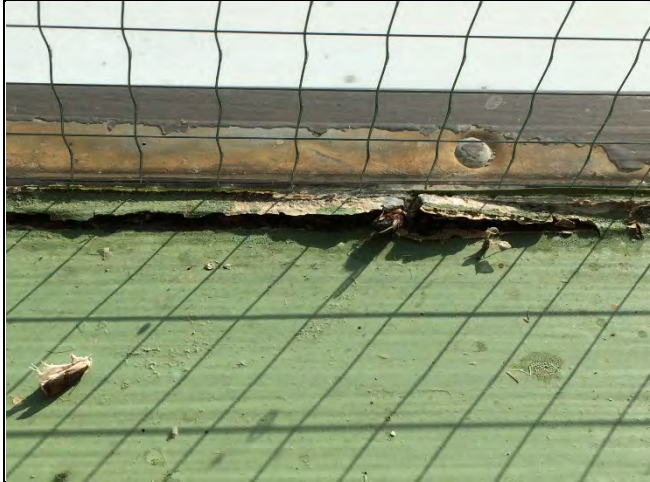
Photo 1: Asbestos-containing interior glazing compound – white was observed to be in poor condition at the west stairwell.
