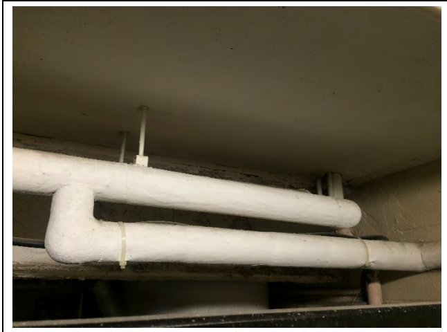
Photo 1: Insulating cement on pipe fittings identified to be asbestos-containing in the first floor garbage room (50% Chrysotile).
