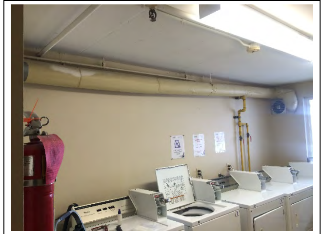
Photo 2: Corrugated paper-like straight pipe insulation identified to be asbestos-containing in the first floor laundry room (65% Chrysotile).
