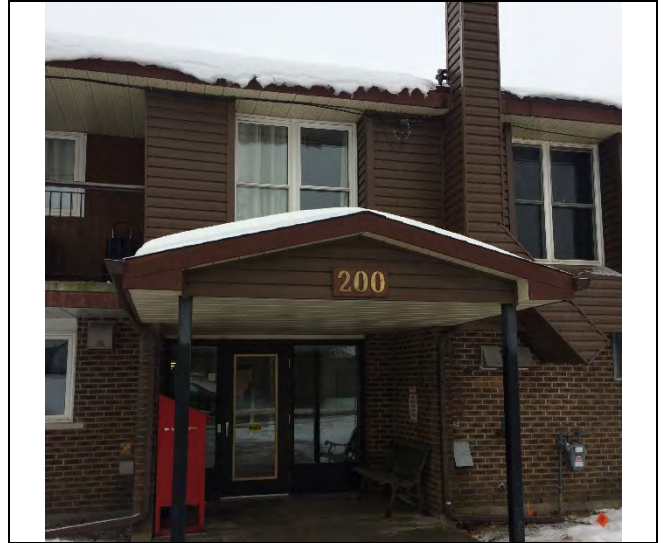
Photo 6: Presumed asbestos-containing brick mortar on exterior walls.
