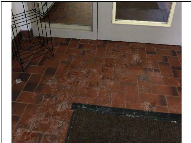
Photo 7: Presumed asbestos-containing ceramic tile grout and mortar/adhesive at the lobby and main entrance.
