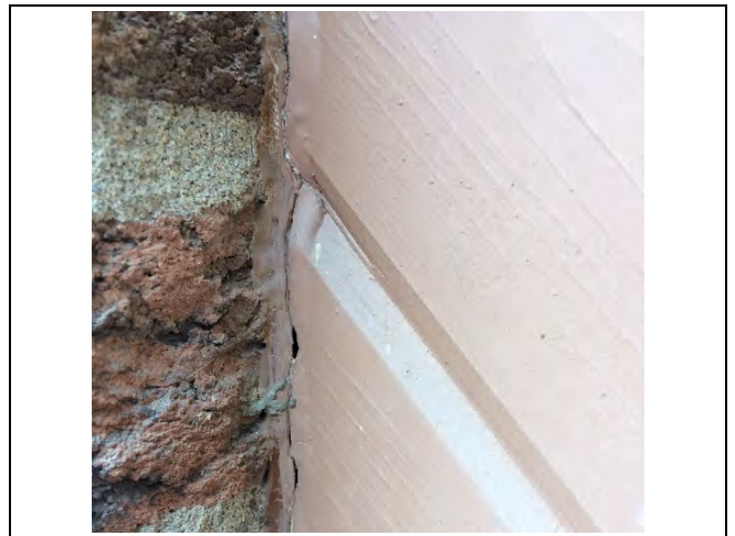
Photo 8: Presumed asbestos-containing exterior caulking – brown on the joint of the walls around the window of the lounge room.
