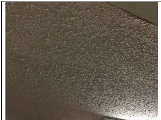
Photo 3: Asbestos-containing stucco – medium rough pattern (1% Chrysotile) on the ceiling in the 1 st floor south stairwell.
