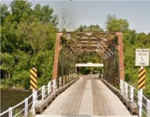
Very Poor Bridge (Andrewsville)
