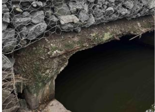
Poor Culvert (East Cardinal Creek)
