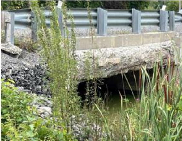
Poor Bridge (Sparks)
