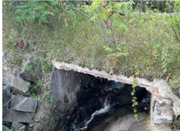
Very Poor Culvert (Leeder)
