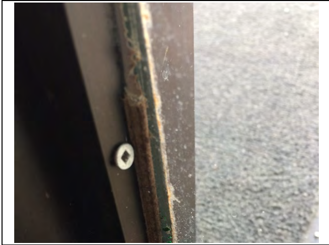
Photo 5: Asbestos-containing interior / exterior glazing compound – grey (4.42% Chrysotile) at the main entrance window.
