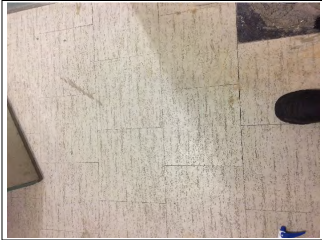
Photo 1: Asbestos-containing 12"x12" vinyl floor tiles – beige with black spots (3.89% Chrysotile) in the communal storage room.
