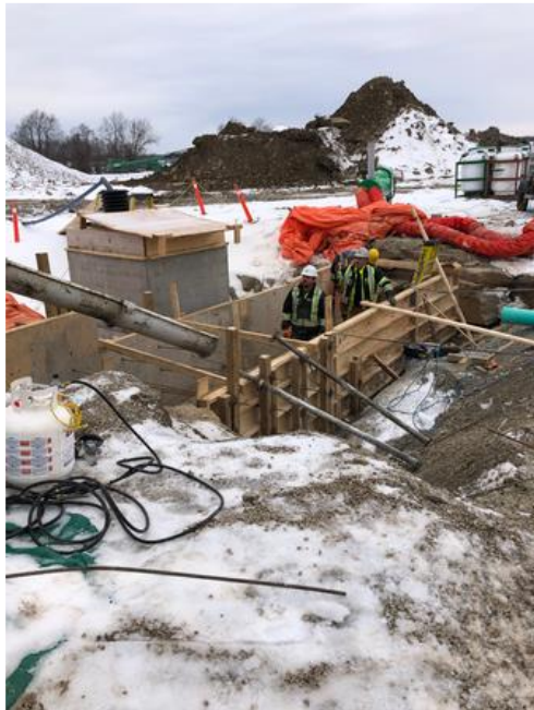
Lean mix concrete formed and poured for footing at fire pit tank
