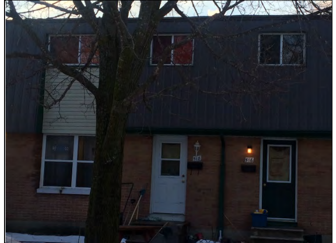
Photo 6: Presumed asbestos-containing brick mortar observed to be present on the exterior walls.
