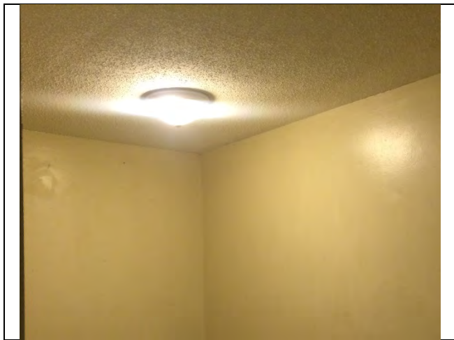
Photo 3: Asbestos-containing drywall joint-fill compound and stucco observed at 550 Fort Town Drive.
