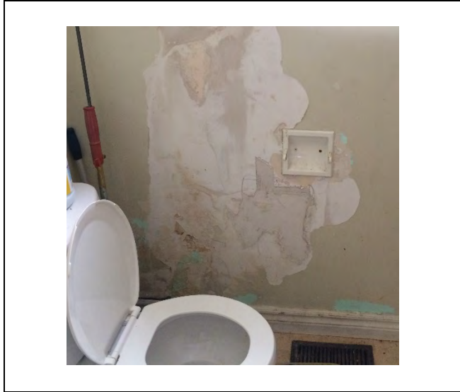
Photo 1: Asbestos-containing drywall joint-fill compound observed to be in poor condition on wall in the washroom at 555 Fort Town Drive.
