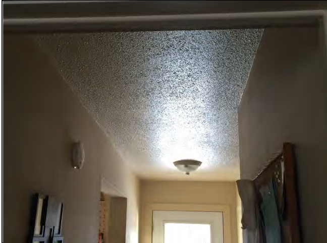
Photo 5: Asbestos-containing stucco and drywall joint-fill compound observed at 563 Fort Town Drive.
