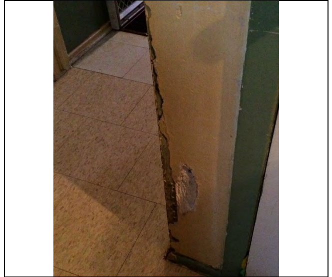
Photo 2: Asbestos-containing drywall joint-fill compound observed to be in poor condition on the kitchen wall at 574 Fort Town Drive.
