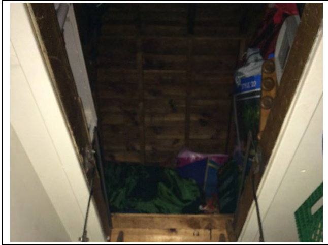
Photo 1: Asbestos-containing drywall joint-fill compound was observed to be in good condition on the walls and ceiling in the storage room access to the attic.
