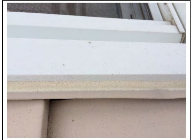
Photo 2: Presumed asbestos-containing exterior caulking – white on the exterior window.
