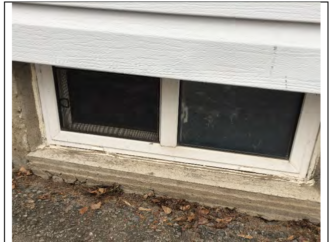
Photo 4: Presumed asbestos-containing exterior caulking – white was observed on the exterior window.
