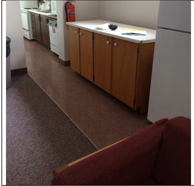
Photo 5: Presumed asbestos-containing mastic associated with 12"x12" vinyl floor tiles – pink mosaic pattern.
