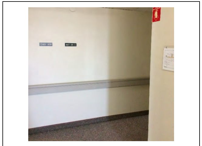
Photo 4: Asbestos-containing drywall joint-fill compound in the 8 th floor corridor near the elevator lobby.
