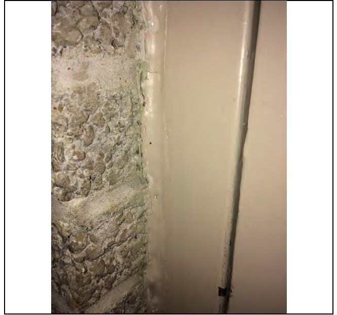
Photo 6: Presumed asbestos-containing brick mortar and exterior door caulking – white (under beige paint) at the back entrance near the elevator door.
