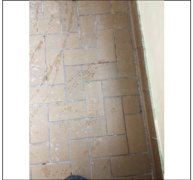
Photo 2: Presumed to be asbestos-containing ceramic tile grout and mortar/adhesive in the lobby.
