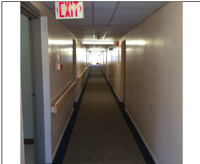
Photo 3: Drywall joint-fill compound identified to be asbestos-containing in the hallways (1% Chrysotile).
