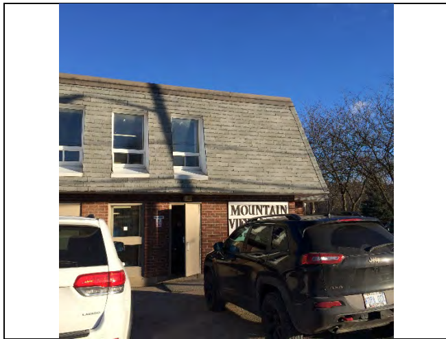
Photo 7: Exterior window and door caulking is presumed to be asbestos-containing.
