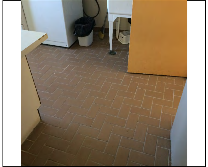
Photo 6: Ceramic tile grout and mortar/adhesive is presumed to be asbestos-containing in the laundry room.
