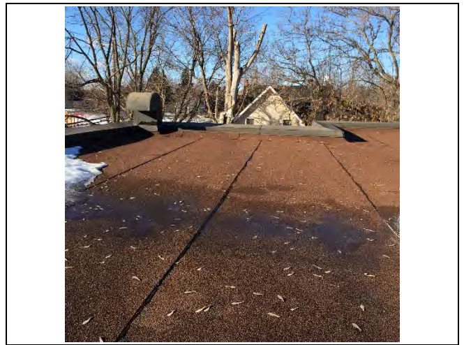
Photo 8: Roof shingles are presumed to be asbestos-containing.
