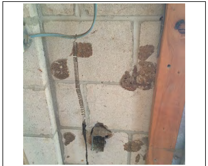
Photo 4: Mastic puck – brown on the block walls in the exterior garage identified to be asbestos-containing (1.2% Chrysotile).
