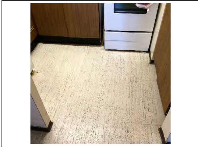
Photo 1: 12"x12" vinyl floor tile – beige with grey specks identified to be asbestos-containing in Unit 101 (1.45% Chrysotile).
