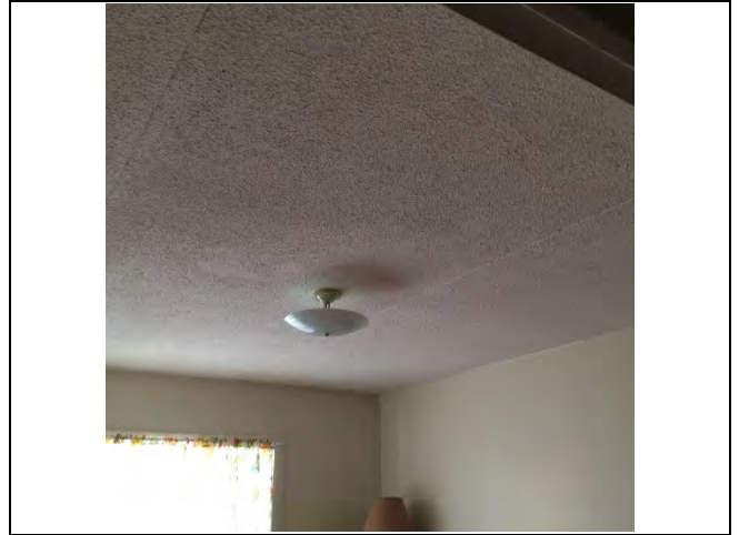
Photo 2: Stucco identified to be asbestos-containing in Unit 210 (3% Chrysotile).
