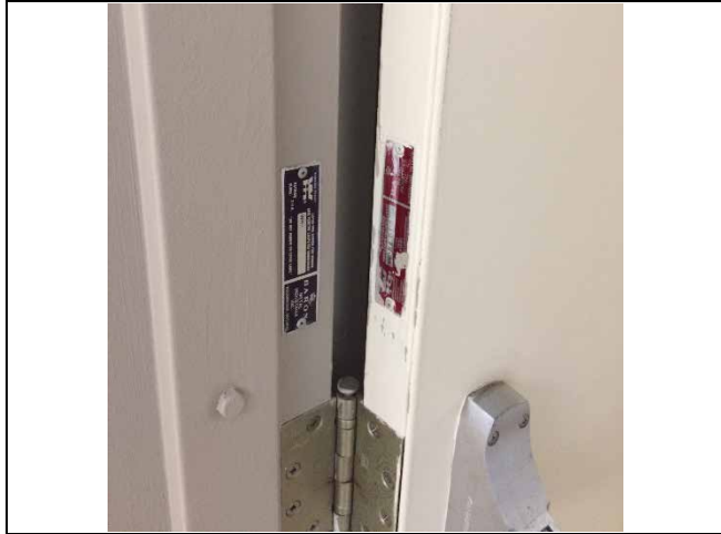
Photo 1: Presumed asbestos-containing fire rated door.
