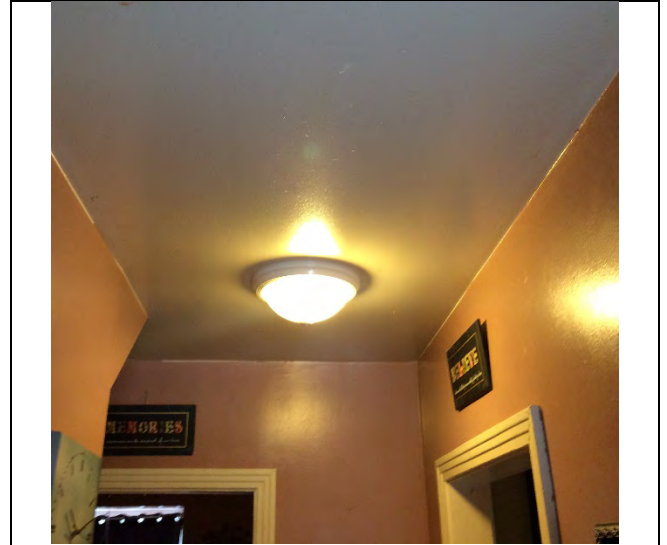
Photo 2: Asbestos-containing drywall joint-fill compound (1% Chrysotile).
