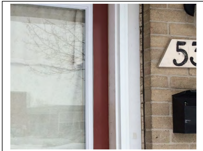
Photo 3: Asbestos-containing exterior door caulking – black (3.1% Chrysotile).
