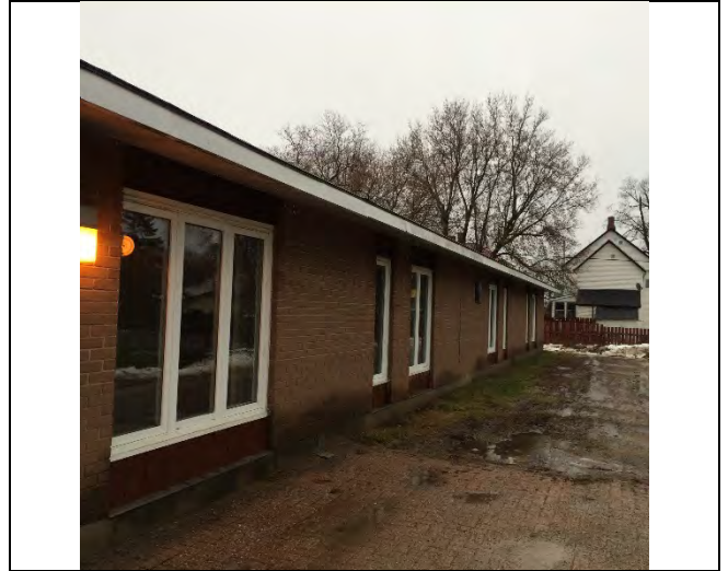
Photo 6: Exterior window caulking – white is presumed to be asbestos-containing.
