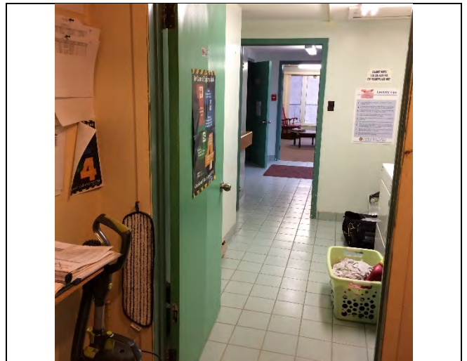
Photo 8: Fire rated door – wood is presumed to be asbestos-containing.
