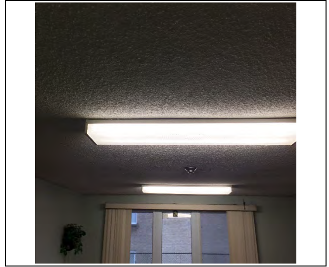
Photo 2: Stucco on ceilings is identified to be asbestos-containing (3% Chrysotile).
