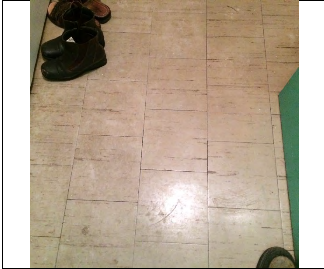
Photo 1: 9"x9" vinyl floor tile – grey with brown streaks is identified to be asbestos-containing (1.52% Chrysotile).
