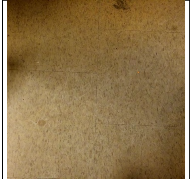
Photo 2: 12"x12" vinyl floor tile – beige with grey specks identified to be asbestos-containing in Unit 207 (2.22% Chrysotile).
