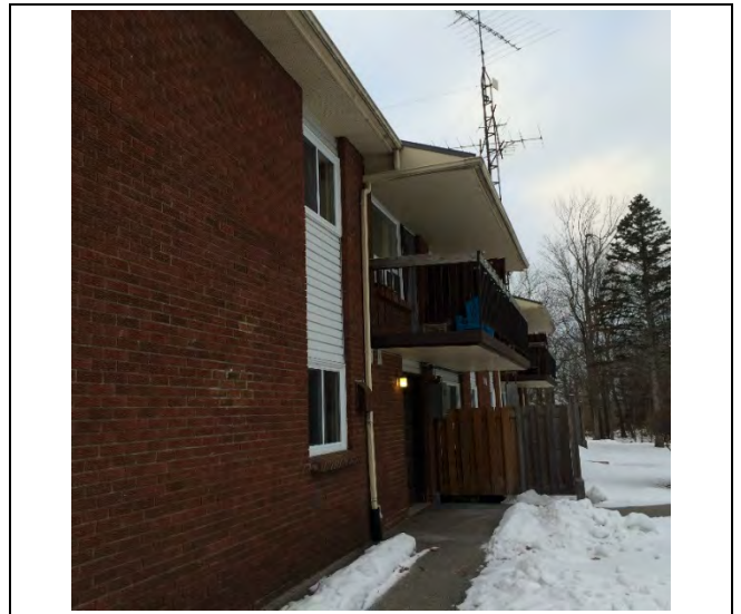
Photo 4: Brick mortar presumed to be asbestos-containing.
