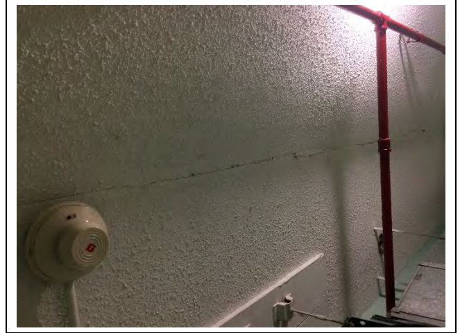
Photo 2: Asbestos-containing texture material observed to be cracking in the 2 nd floor laundry room ceiling.
