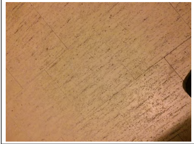
Photo 1: Asbestos-containing 12" x 12" vinyl floor tiles – beige with dots observed to be in good condition in the foyer of unit 107.
