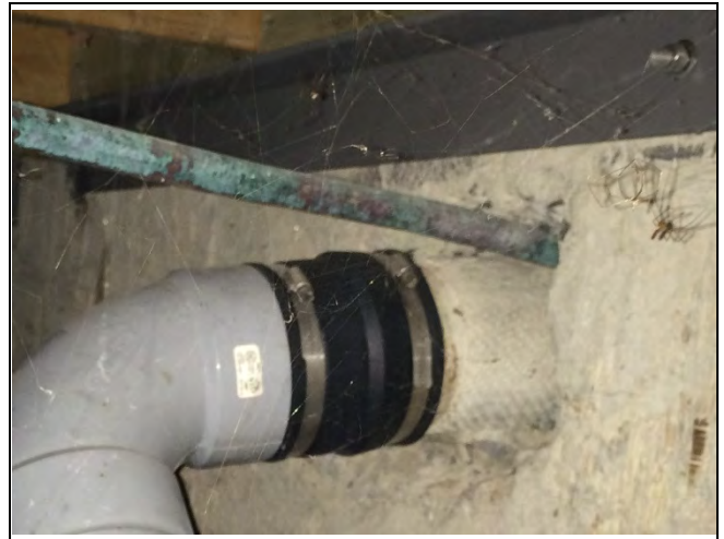
Photo 4: Presumed asbestos-containing cement pipe observed to be in good condition in the crawlspace.
