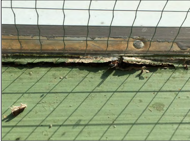
Photo 1: Asbestos-containing interior glazing compound – white was observed to be in poor condition at the west stairwell.
