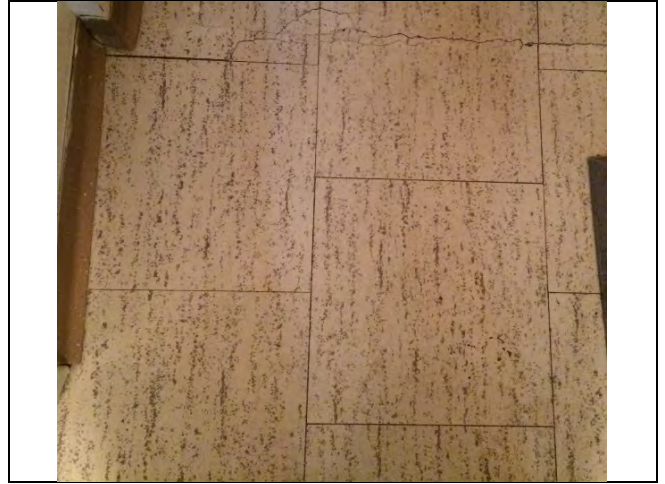
Photo 2: Asbestos-containing 12"x12" vinyl floor tile – beige with grey specks was observed in unit 209 hallway.
