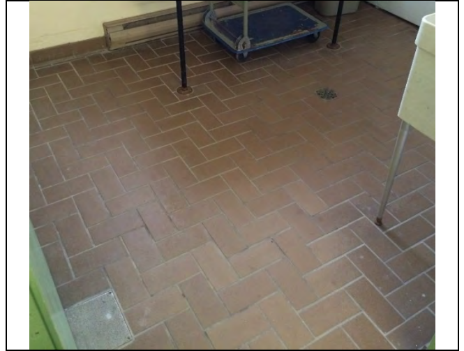
Photo 6: Presumed asbestos-containing ceramic tile grout and mortar / adhesive was observed in the 1 st floor laundry room.
