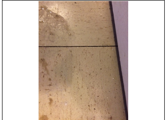
Photo 6: Asbestos-containing 12"x12" vinyl floor tiles – beige with black flecks observed to be in good condition on the basement landing at 280 Bartholomew Street Unit #8.
