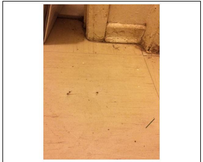
Photo 4: Asbestos-containing 12"x12" vinyl floor tiles – beige with brown streaks observed to be in good condition on the basement landing at 280 Bartholomew Street Unit #4.
