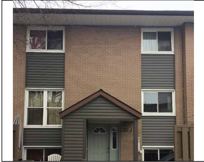
Photo 1: Presumed asbestos-containing brick mortar observed to be in good condition on the exterior walls at 280 Bartholomew Street Unit #4.
