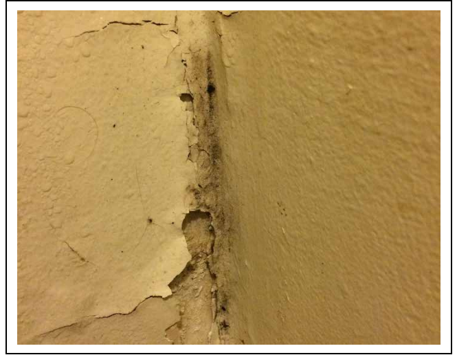
Photo 2: Asbestos-containing drywall joint-fill compound observed to be in poor condition on the wall in the foyer at 280 Bartholomew Street Unit #4.
