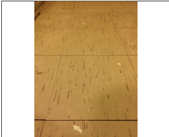
Photo 3: Asbestos-containing 12"x12" vinyl floor tiles – brown with brown streaks observed to be in good condition on the upper level landing at 280 Bartholomew Street Unit #4.
