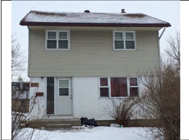
Photo 1: Asbestos-containing exterior texture coat on exterior of house.
