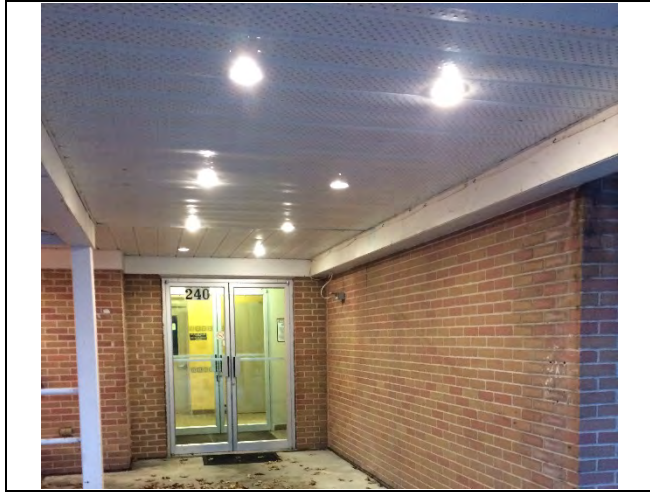
Photo 5: Presumed asbestos-containing brick mortar observed to be in good condition on the exterior walls
