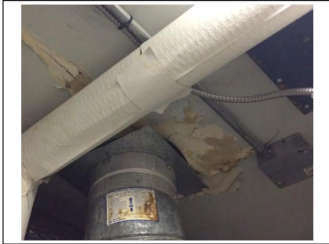
Photo 1: Asbestos-containing drywall joint-fill compound observed to be in poor condition on the ceiling in the hot water tank room located in the laundry room.
