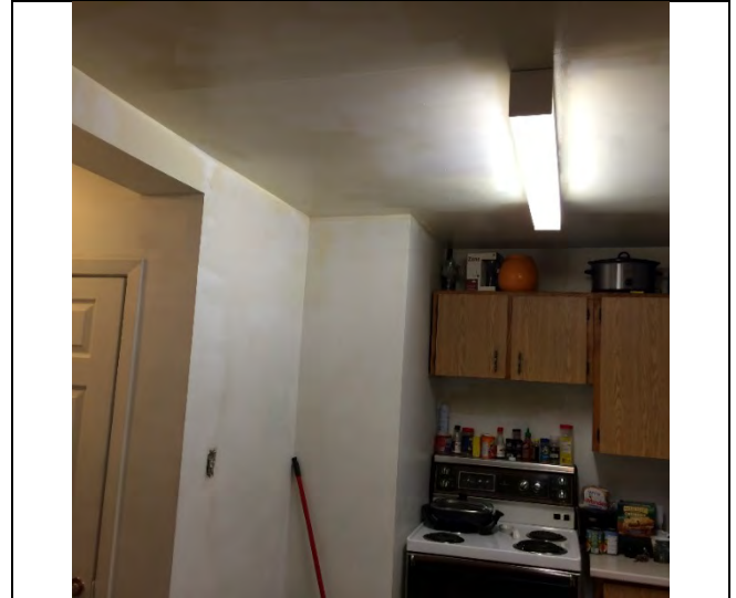
Photo 2: Asbestos-containing drywall joint-fill compound was observed on walls and ceiling.
