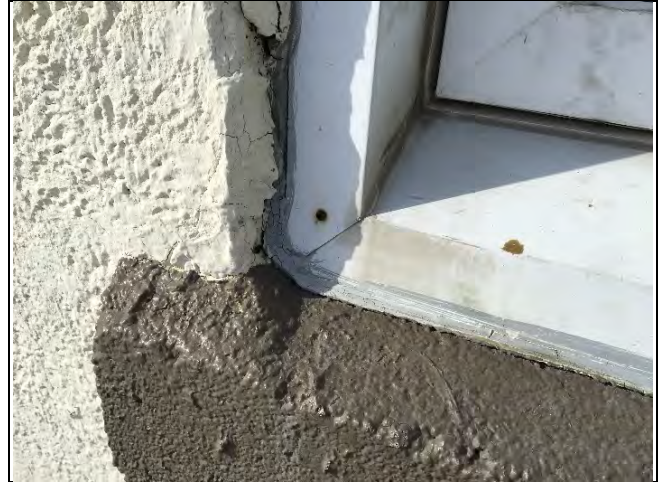
Photo 2: Presumed asbestos-containing exterior window caulking – grey observed at 203 Prescott Street.
