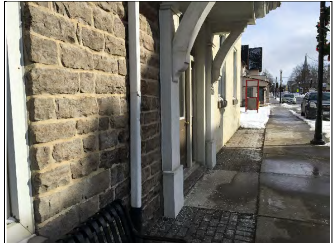
Photo 4: Presumed asbestos-containing brick mortar observed at the exterior of 201 Prescott Street.
