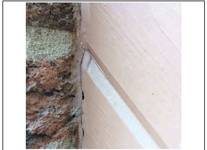
Photo 8: Presumed asbestos-containing exterior caulking – brown on the joint of the walls around the window of the lounge room.
