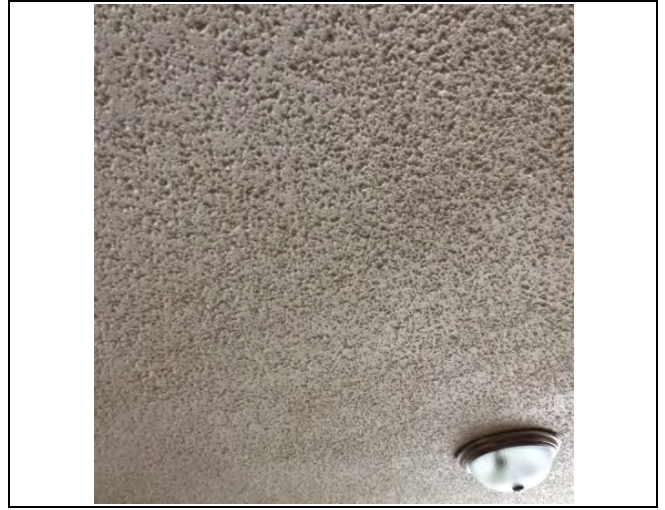
Photo 2: Asbestos-containing stucco - rough pattern (1% Chrysotile) on ceiling in the living room of unit 212.
