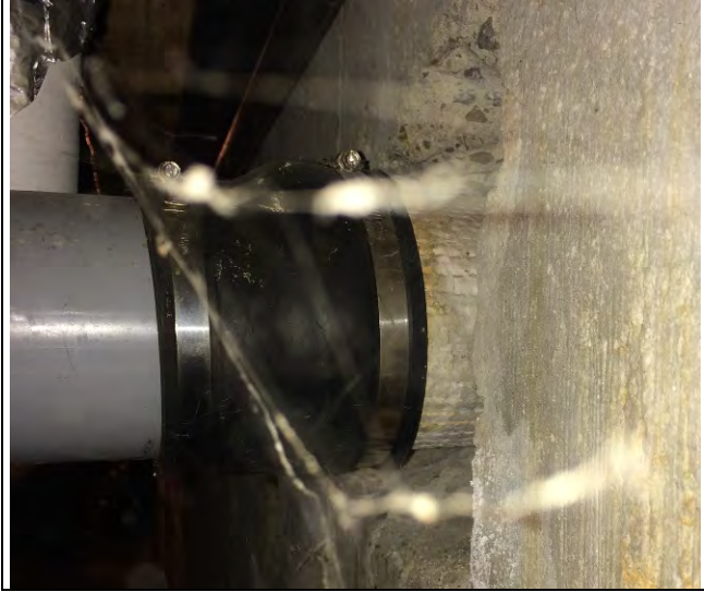
Photo 5: Presumed asbestos-containing cement pipe in the crawlspace.
