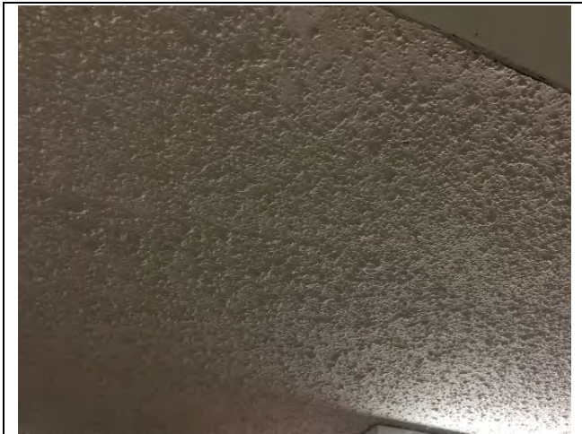
Photo 3: Asbestos-containing stucco - medium rough pattern (1% Chrysotile) on the ceiling in the 1 st floor south stairwell.
