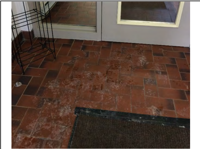
Photo 7: Presumed asbestos-containing ceramic tile grout and mortar/adhesive at the lobby and main entrance.
