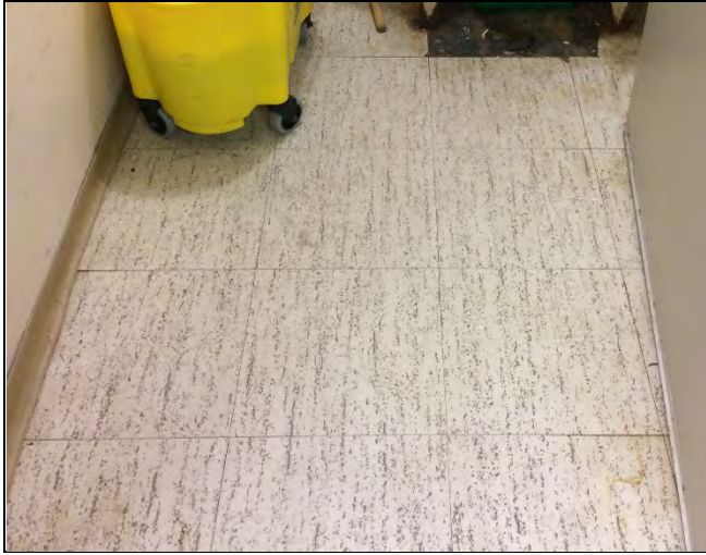
Photo 1: Asbestos-containing 12" x 12" vinyl floor tiles beige with black dots (2.41% Chrysotile) and associated mastic (0.95% Chrysotile) observed in the custodian's closet. The mastic was exposed at the right corner.
