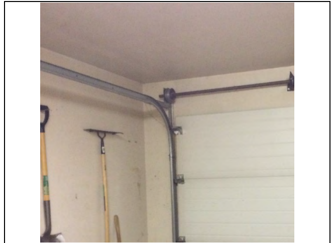
Photo 4: Asbestos-containing drywall joint-fill compound (1% Chrysotile) on the walls and ceiling in the garage.
