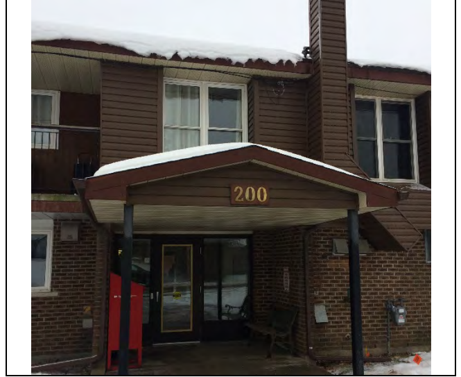
Photo 6: Presumed asbestos-containing brick mortar on exterior walls.
