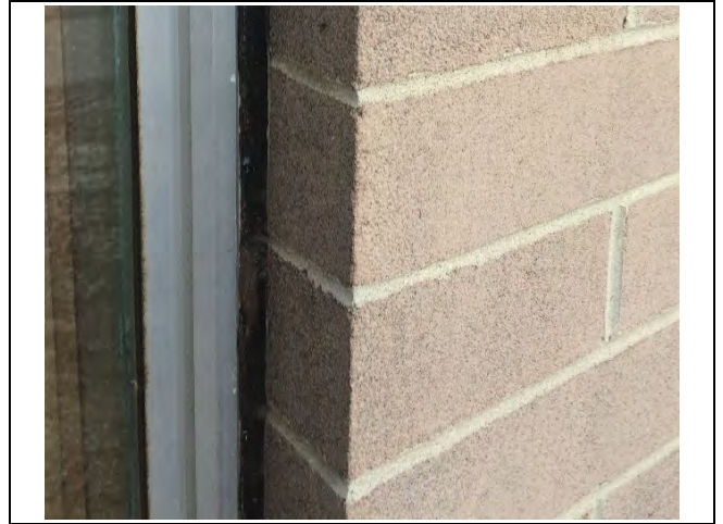
Photo 2: Asbestos-containing exterior window caulking – black (0.85% Chrysotile) near the main entrance.
