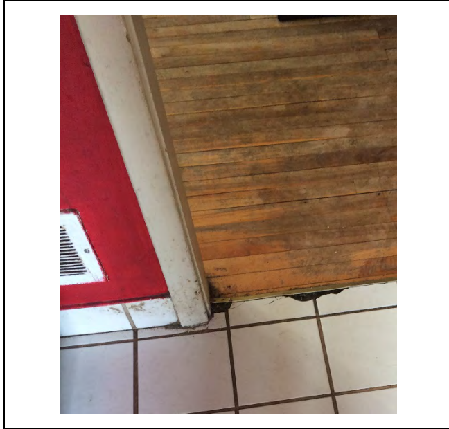
Photo 1: Asbestos-containing drywall joint-fill compound on the kitchen walls and presumed asbestos-containing ceramic tile grout and mortar / adhesive on the kitchen floor.
